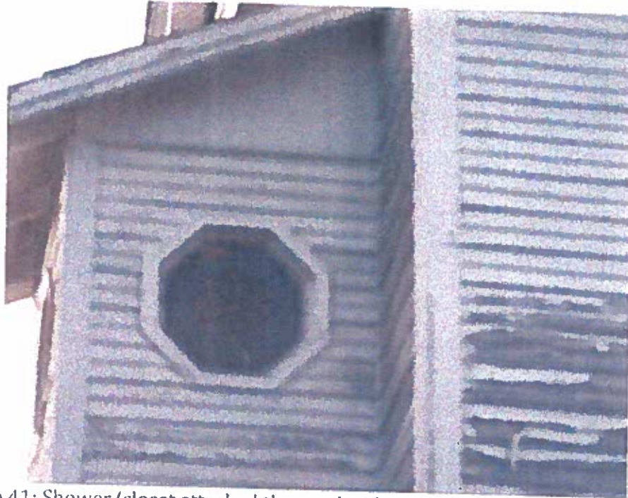
Photo 41: Shower/closet attached the south side of 2 nd floor. View from the east. The window is fixed and can not be opened.
