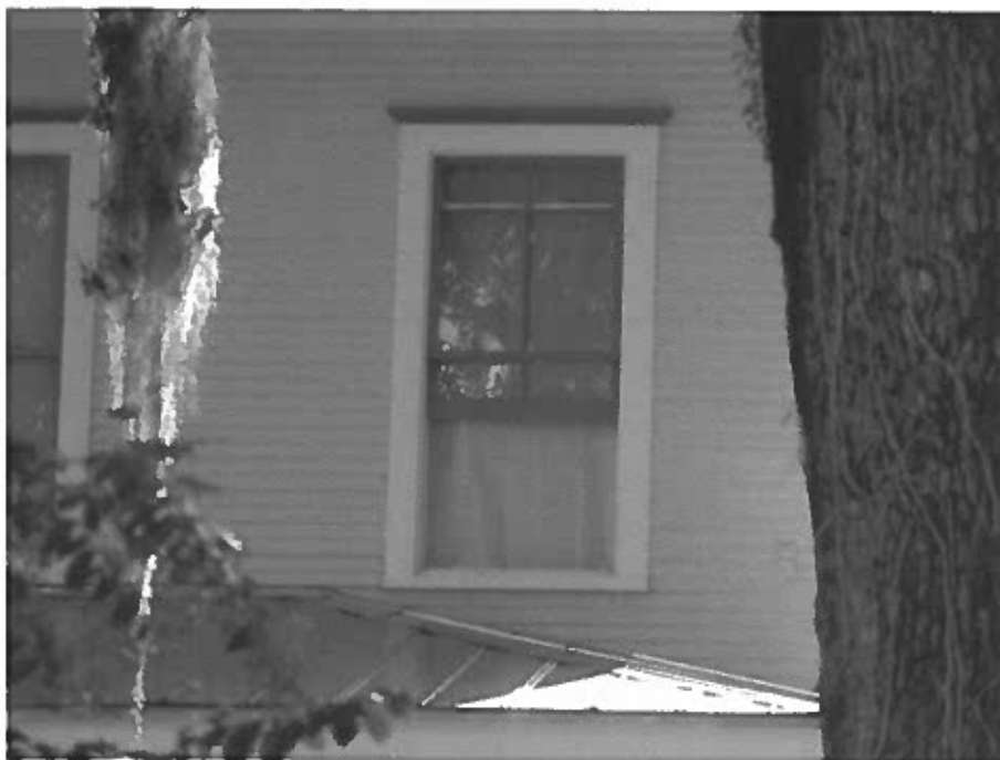
Photo 49: 2 nd floor window to the northwest room facing north (to the right of the window shown in Photo 48). The window was partially operational but missing hardware. Now restored and operational.
