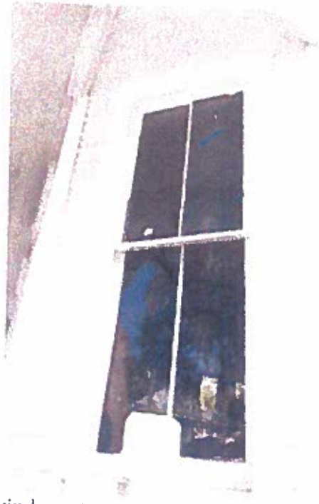
Photo 27: 1 st floor window at western end of porch. Window is painted shut and may not be operable.
