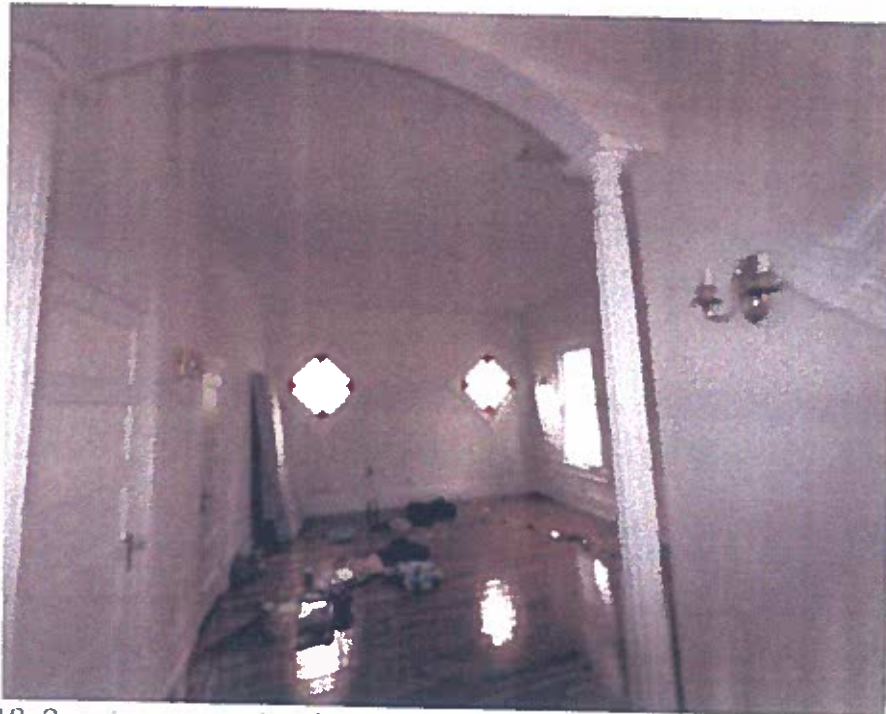
Photo 18: Opening connecting the two 2 nd floor rooms at the north side of the house.
