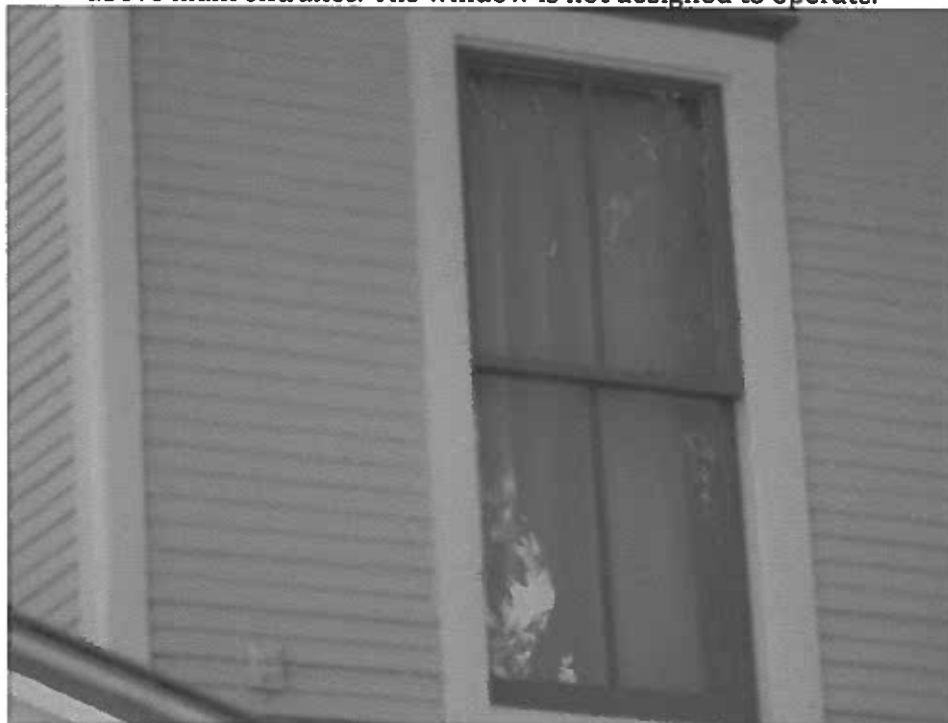
Photo 48: 2 nd floor northwest room facing south. This window was partially operational but some hardware was missing. Now restored and operational (to the left of the window shown in Photo 49).
