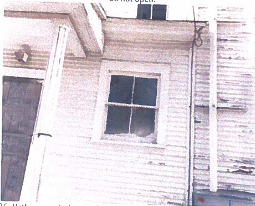
Photo 36: Bathroom window to the right of the kitchen door. The window has been replaced, but some original trim remains.
