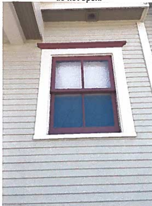
Photo 36: Bathroom window to the right of the kitchen door. The window has been replaced, but some original trim remains.
