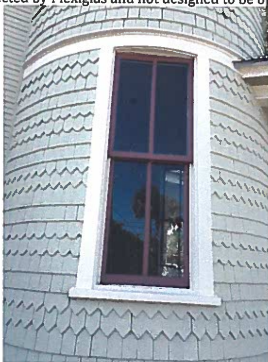
Photo 34: 1 st floor window facing east. This window is part of the turret at the north-east corner.
