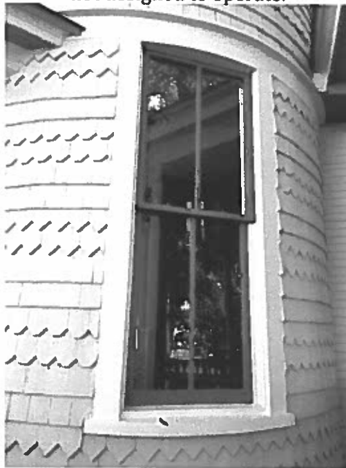
Photo 32: Window to the left of entrance door, facing approx.. north. Window panes appear modern. Was paint shut, now operational
