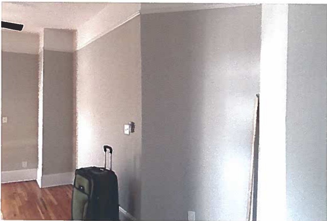
Picture 16: Upstairs hallway facing the angled wall connecting the east bathroom and the south east bedroom.
