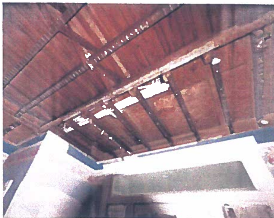
Picture 10: South-West room ceiling
