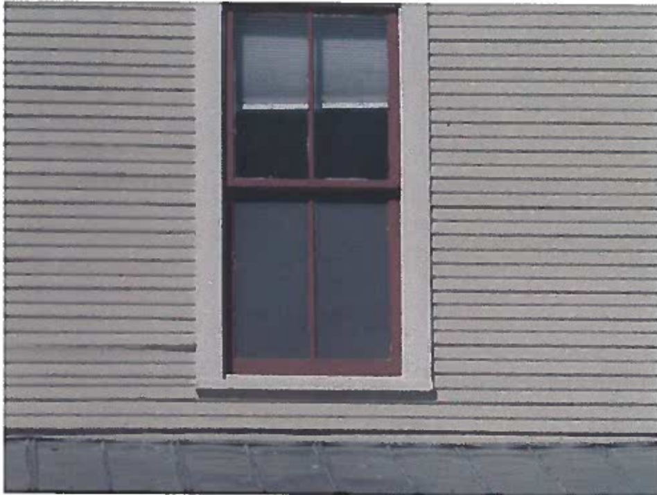
Photo 39: 2 nd floor southwest bedroom window facing south. The window has been paint shut now operational.
