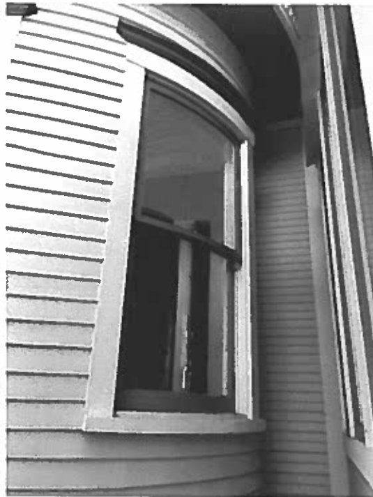
Photo 31: Curved Window on west-side turret facing south. Window is paint shut / not designed to operate.
