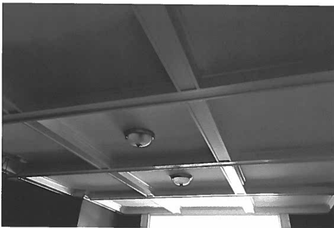
Picture 10: South-West room ceiling
