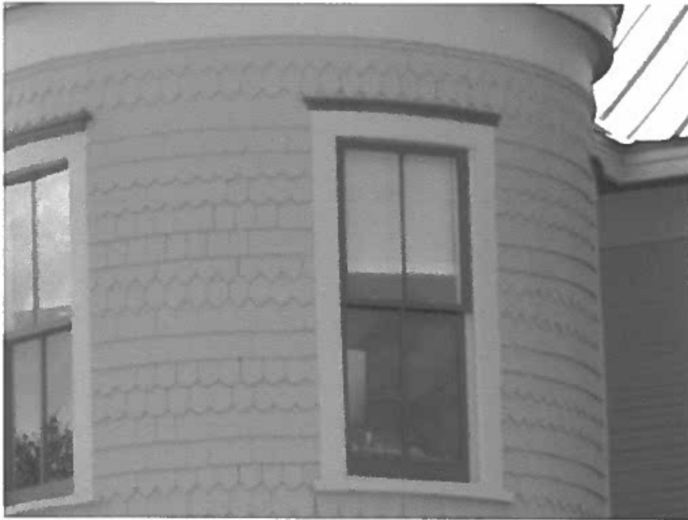
Photo 45: Window of 2 nd floor turret facing northeast. Panes were broken and window was pain shut. Now restored and operational.
