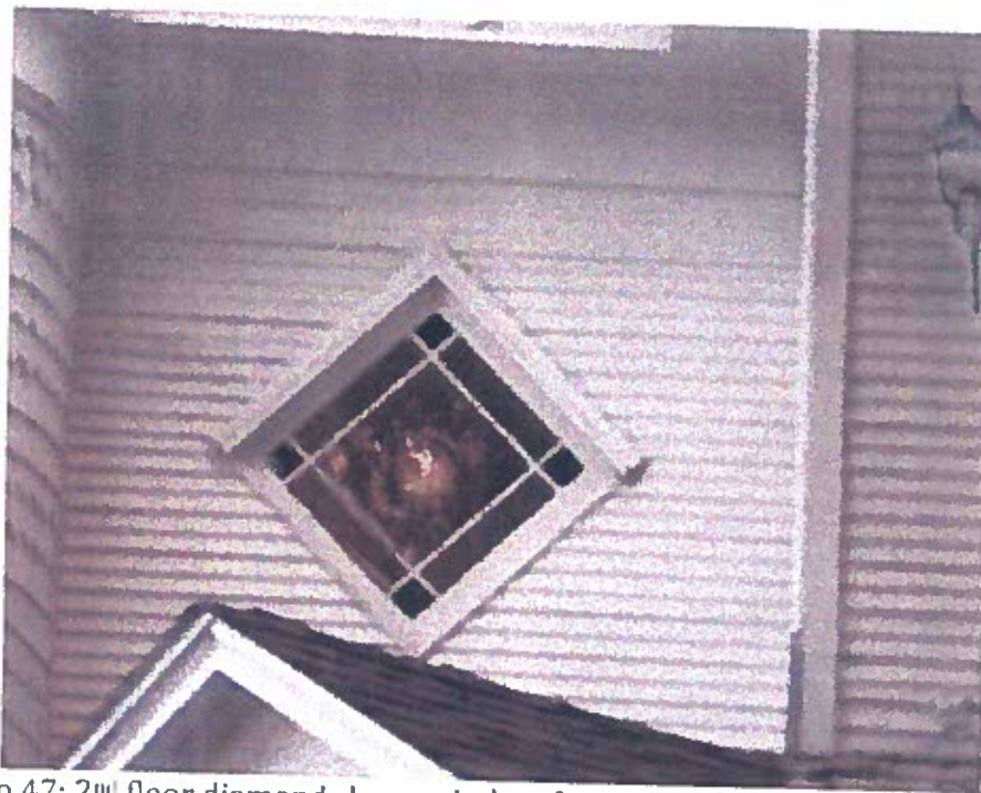
Photo 47: 2 nd floor diamond shape window facing north right next to the turret above main entrance. The window is not designed to operate.
