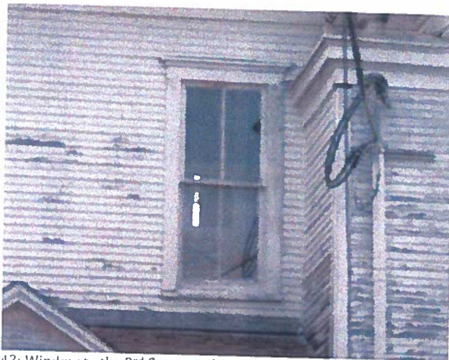
Photo 43: Window to the 2 nd floor east bathroom. Glass broken, window currently not operable.
