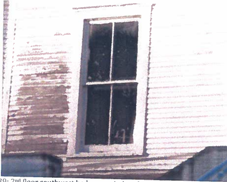
Photo 39: 2 nd floor southwest bedroom window facing south. The window has been paint shut and may or may not operate.
