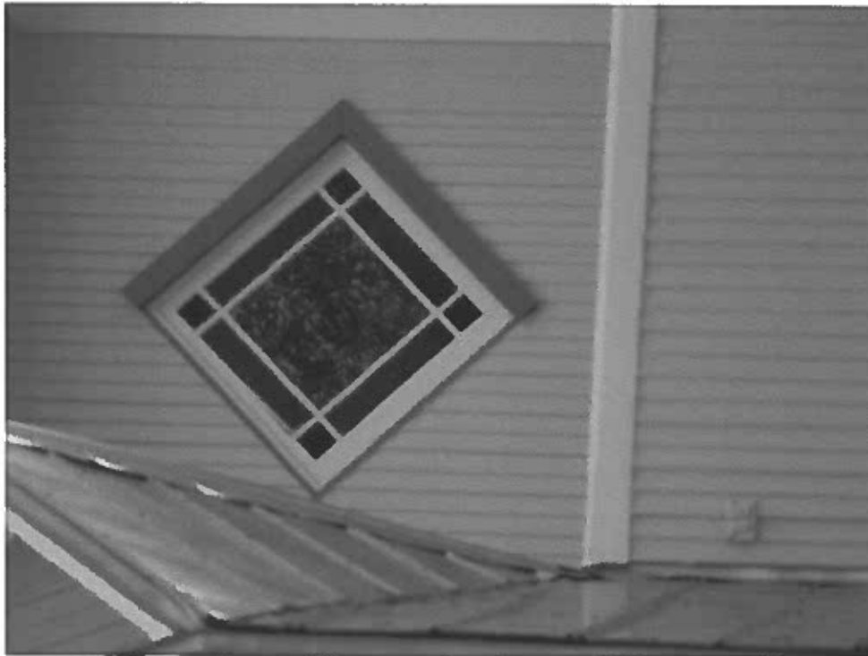
Photo 47: 2 nd floor diamond shape window facing north right next to the turret above main entrance. The window is not designed to operate.
