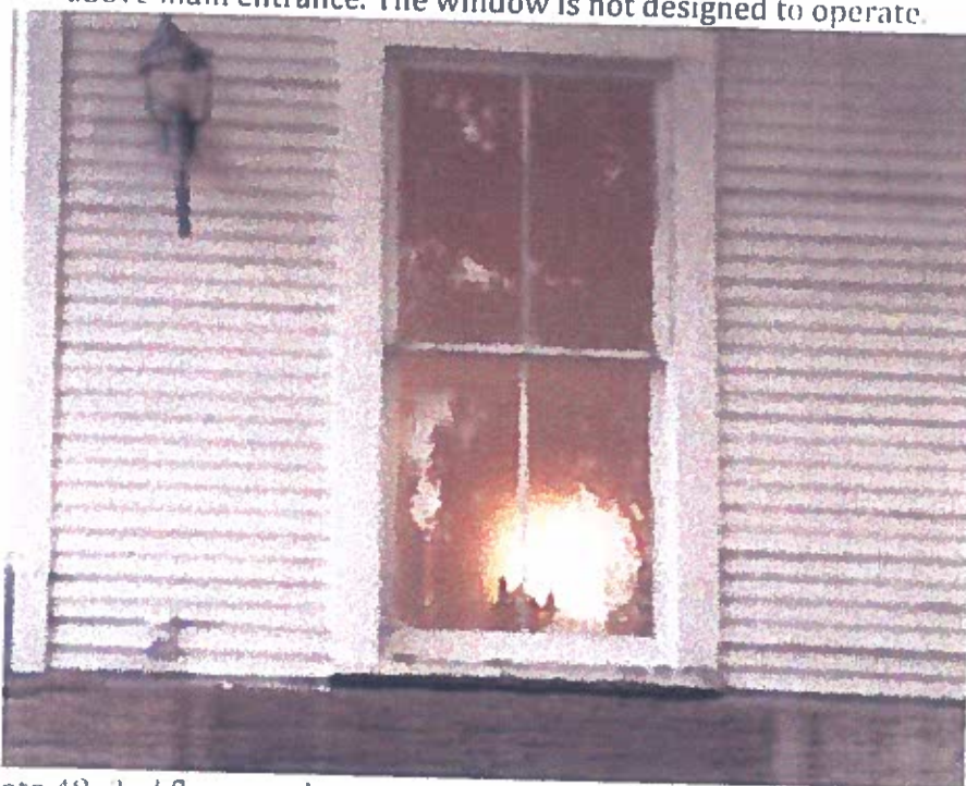
Photo 48: 2 nd floor northwest room facing south. This window is partially operational but some hardware is missing. (to the left of the window shown in Photo 49).
