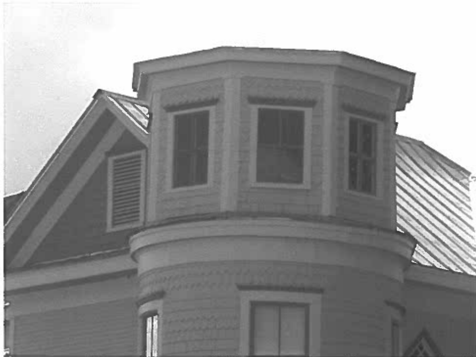
Photo 53: Windows of the turret facing the corner of Market Street and 4 th Street (northeast corner of house). These window open to the attic and are not operational.
