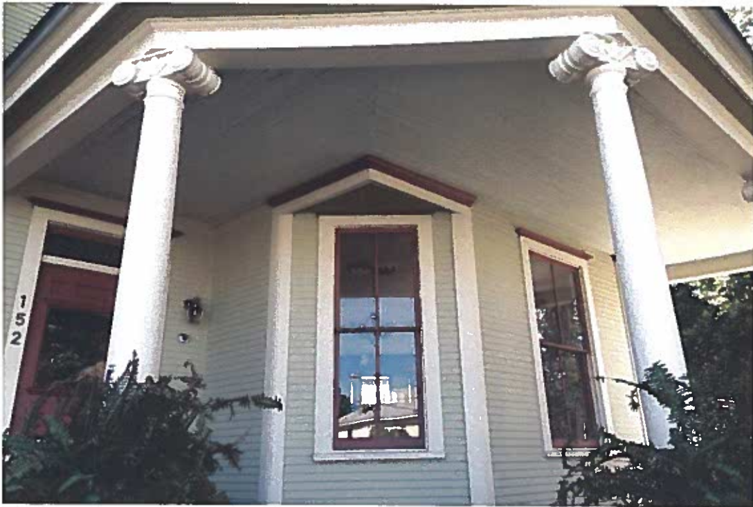
Photo 25: was painted shut window west of entrance, now restored and fully operational (1 st floor)
