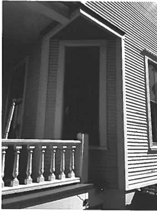
Photo 27: 1 st floor window at western end of porch. Window was painted shut now restored and operational.
