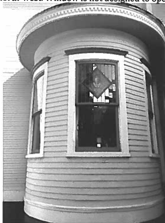
Photo 30: Curved window on west-side turret facing west. Window is paint shut not designed to open.
