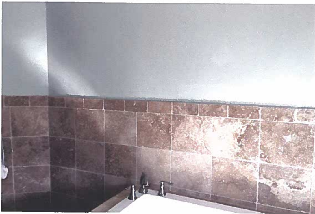
Photo 22: 2 nd Floor was South West bedroom now bathroom. View by Facing east.
