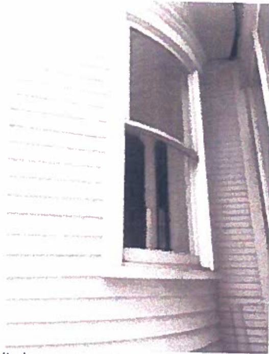
Photo 31: Curved Window on west-side turret facing south. Window is not paint shut / not designed to operate.
