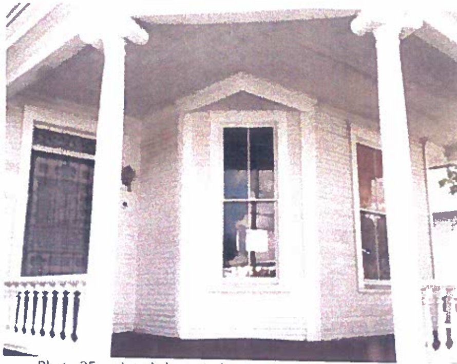
Photo 25: painted shut window west of entrance (1 st floor)
