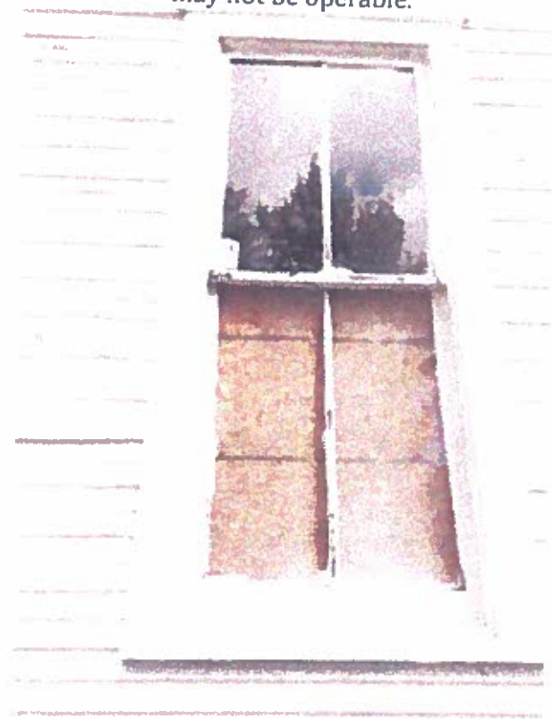
Photo 28: 1 st Floor window facing west. Window may not be operable. Missing panes.
