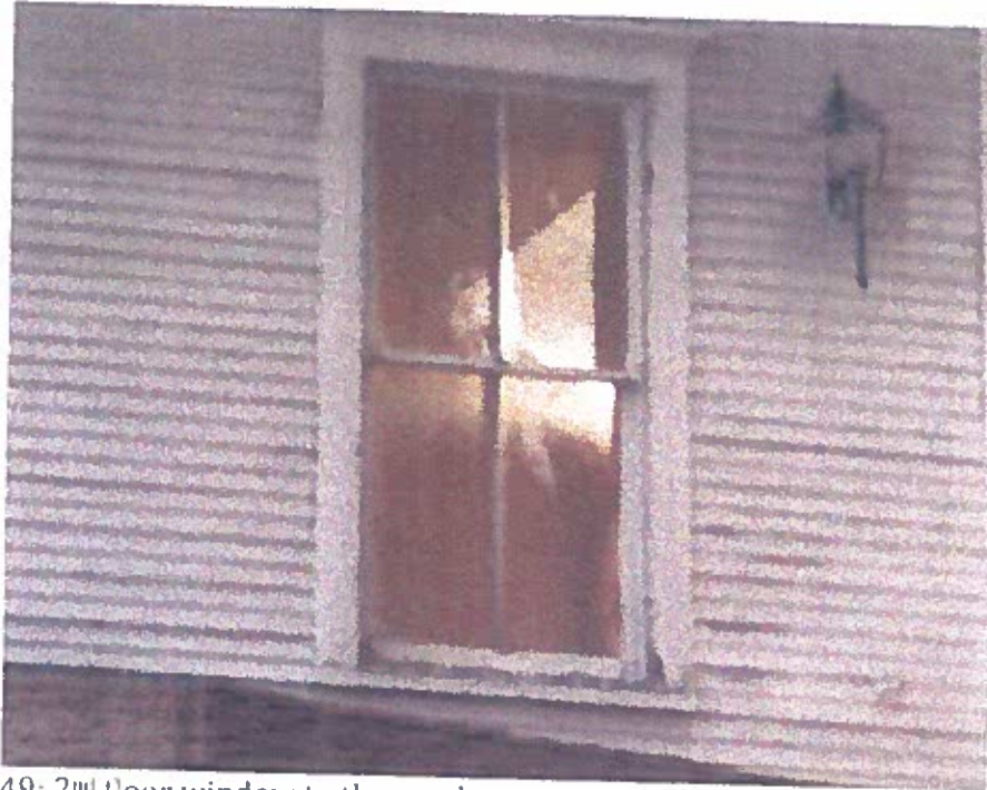
Photo 49: 2 nd floor window to the northwest room facing north (to the right of the window shown in Photo 48). The window is partially operational but missing hardware.
