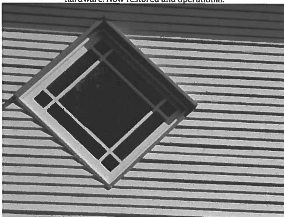
Photo 50: 2 nd floor diamond shape window to the northwest room. This floor is not designed to be opened.
