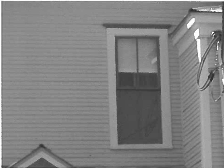
Photo 43: Window to the 2 nd floor east bathroom. Glass was broken, window now restored and operational.
