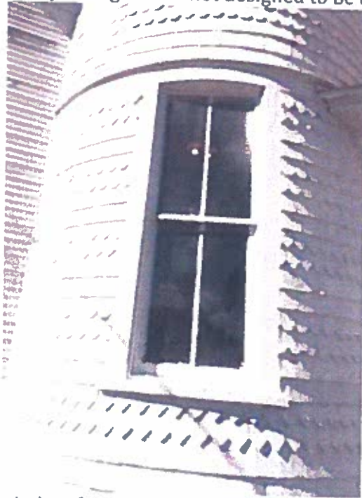
Photo 34: 1 st floor window facing east. This window is part of the turret at the north-east corner.
